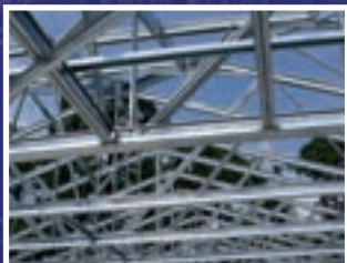
Light Gauge Steel Trusses
